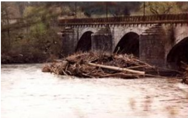
Figure 3. Large woody debris causes problems with undermining the bridges in France. To solve this, wood traps have been built up streams of some of the bridges at risk.
